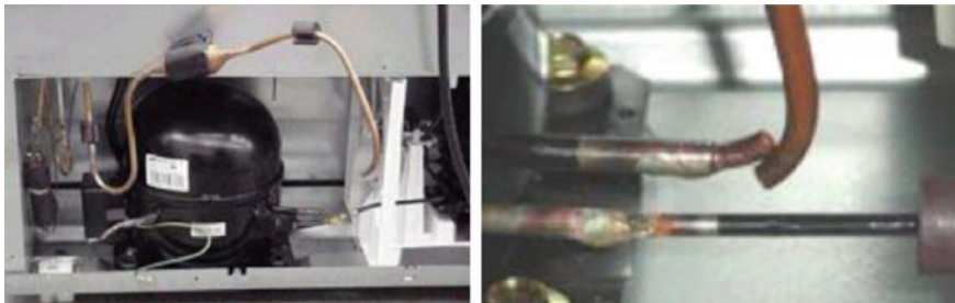
(b) Failed connecting tubes in the mechanical compartment
